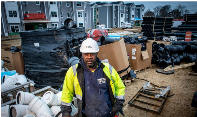
Aaron Vailes works at a construction site in Uniondale. Credit: Newsday / J. Conrad Williams Jr.
